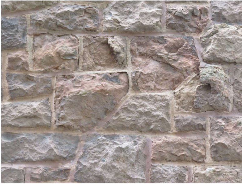
Photo 26: Egleston stone with face delamination.
