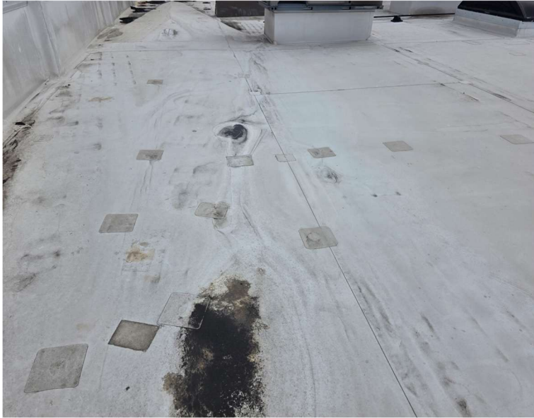
Photo 21: Parish roof with multiple membrane patches.
