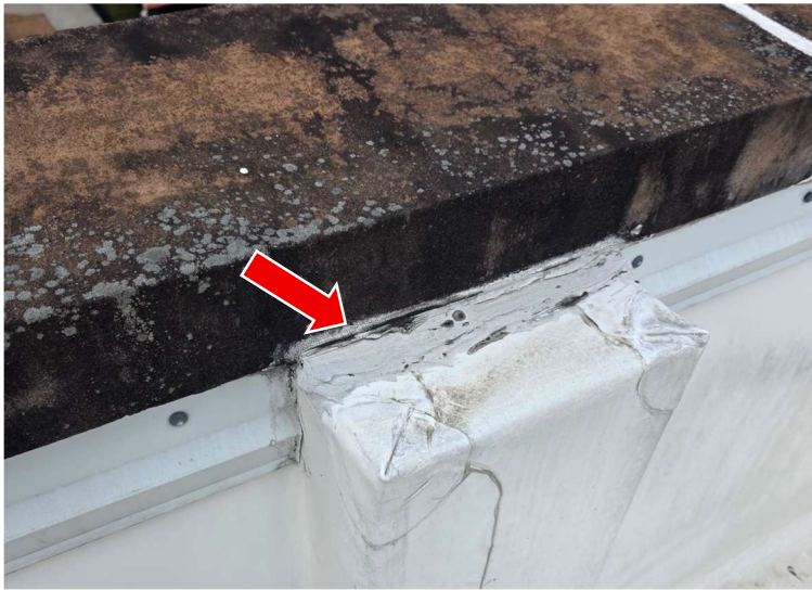
Photo 20: Parish Roof with gaps at sealant.
