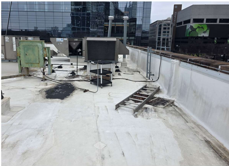
Photo 18: View of Parish House roof with debris accumulation, membrane staining consistent with inadequate drainage.
