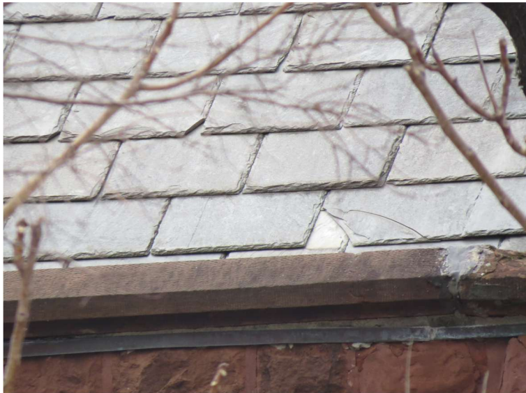
Photo 12: View of Egleston broken slate.
