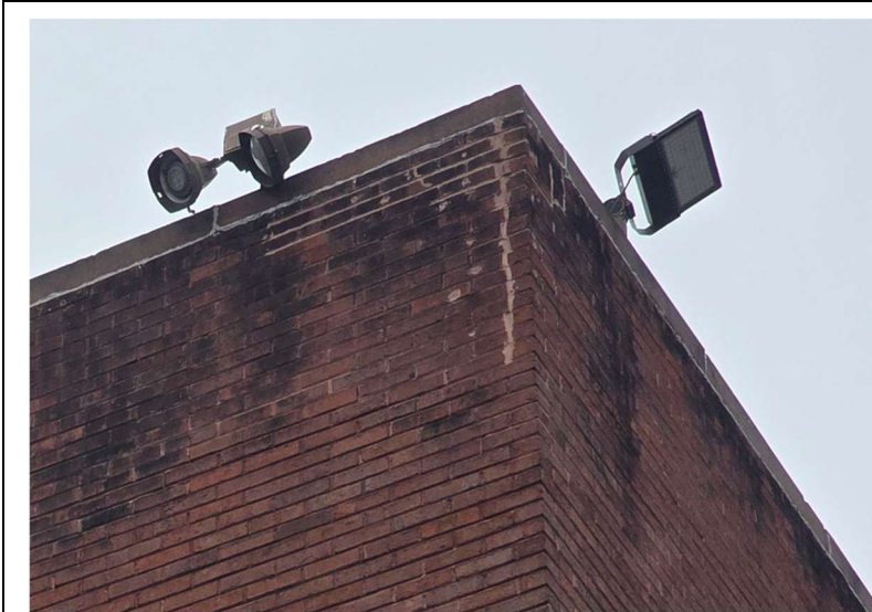
Photo 32: Parish Hall vertical brick crack and repair attempt at corner.
