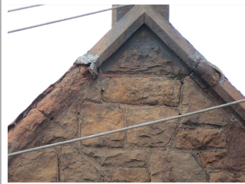
Photo 23: Egleston Hall gable with stone delamination and open stone joints.
