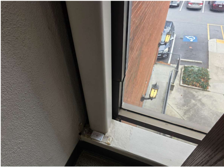
Photo 45: Egleston-Parish connector curtain wall with misaligned sections.
