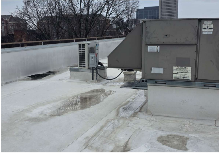
Photo 19: Parish Roof with standing water.
