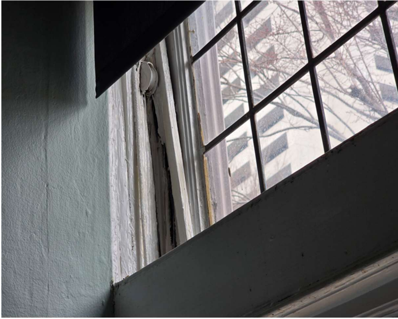
Photo 43: Egleston sash pulley disconnected and sash damage.
