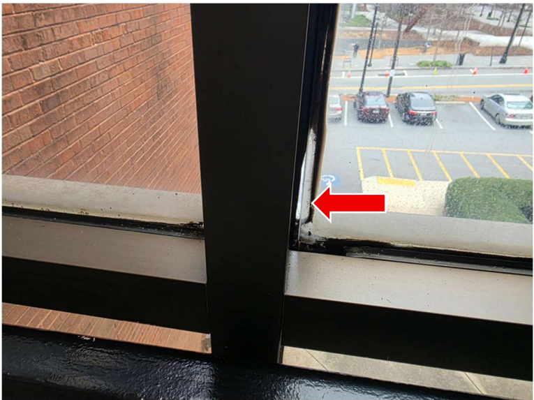
Photo 46: Egleston-Parish connector curtain wall with gap at glazing.
