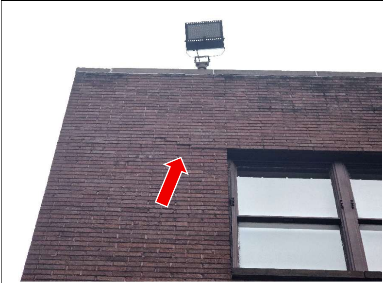
Photo 31: Parish Hall brick bulging.
