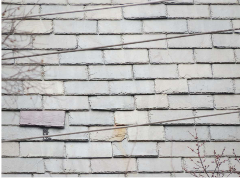
Photo 11: View of Egleston slate with displacement and broken edges.
