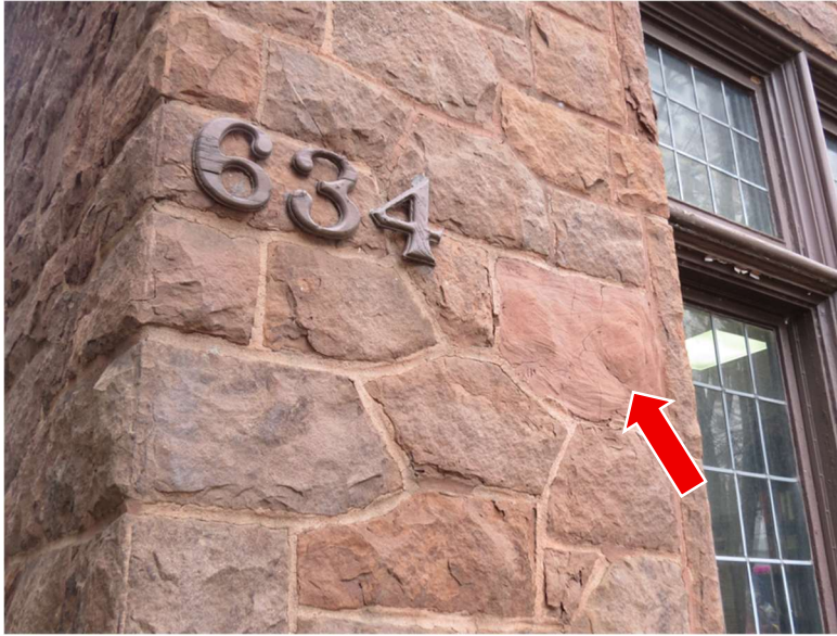
Photo 25: Egleston stone patch with cracks.
