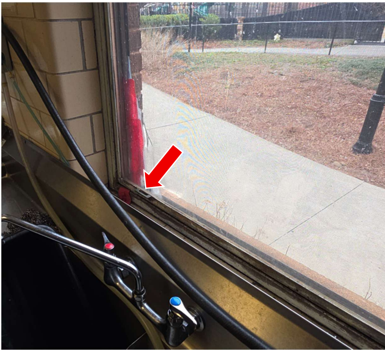
Photo 47: Parish Hall steel sash with gaps at glazing putty.
