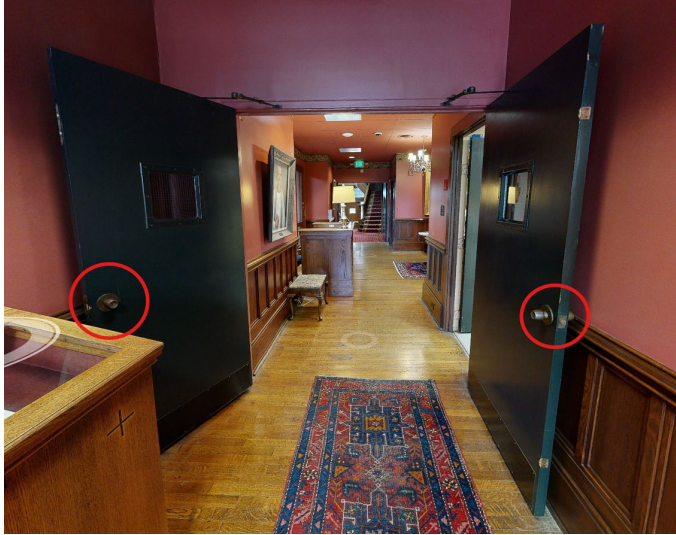
FIGURE 7 EXIT DOOR HARDWARE IS NOT COMPLIANT AND DOOR IS PROPPED OPEN
