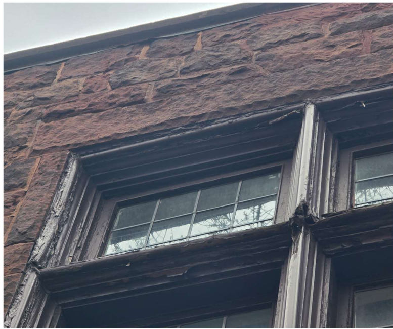
Photo 36: Egleston wood frame decay.
