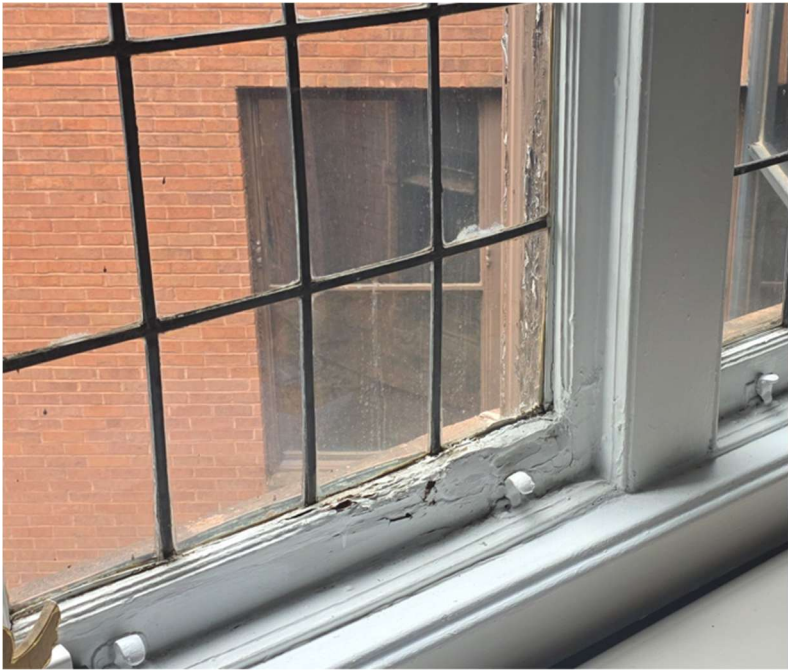
Photo 42: Egleston window sash decay with remedial repair attempts.
