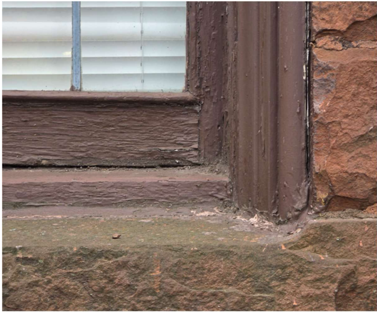
Photo 34: Egleston window frame decay and open joint at brickmold-stone joint.
