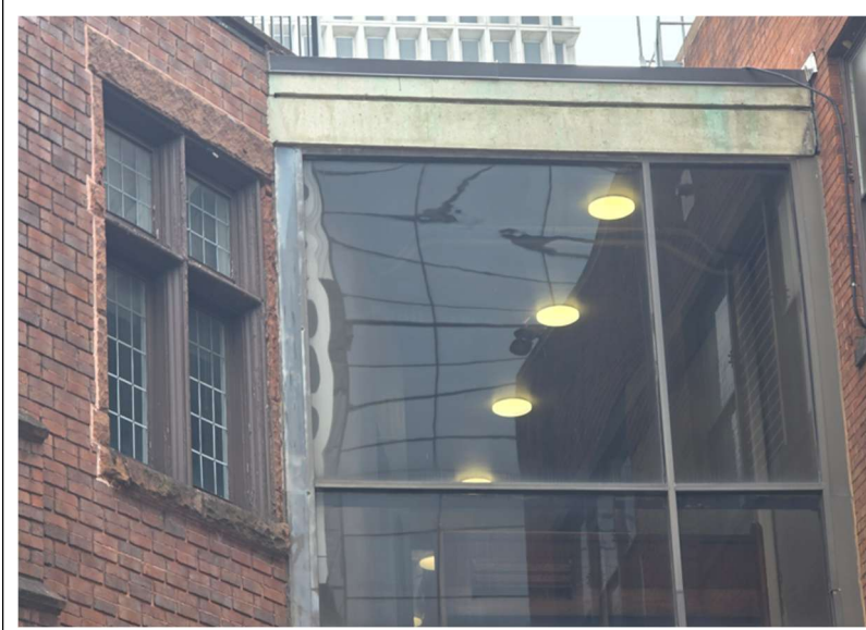
Photo 39: Egleston – Parish connector with deformed glass at curtain wall.
