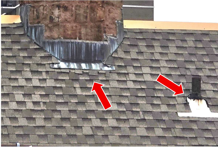
Photo 15: View of Egleston asphaltic shingles with displacement (left), corroded vent pipe (right).
