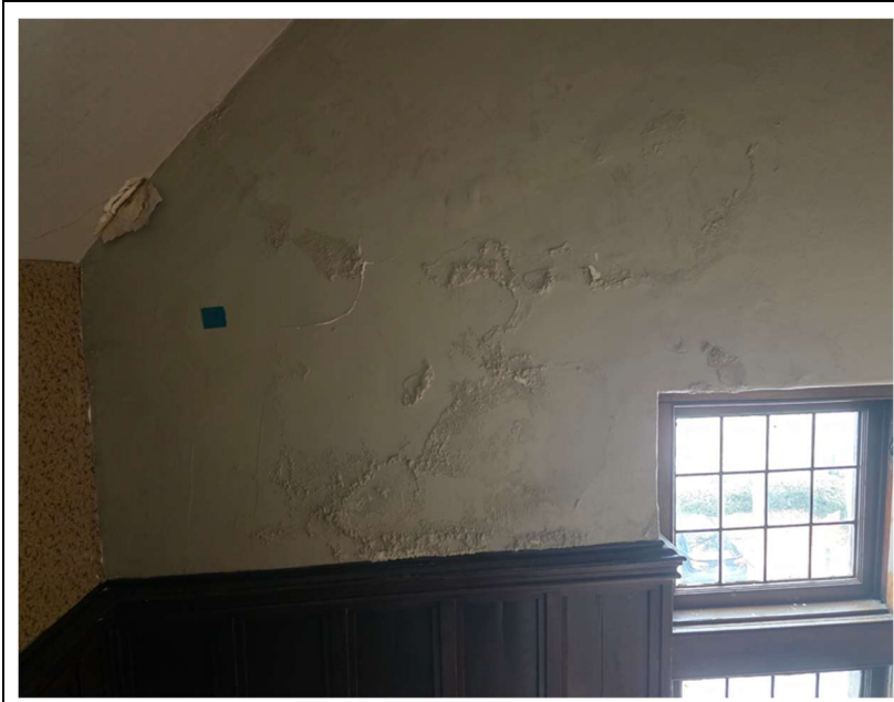
Photo 49: Egleston Hall with plaster damage at gable.
