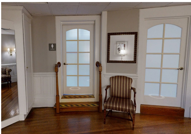
FIGURE 8 RESTROOMS AND BRIDE'S ROOM ARE NOT ACCESSIBLE DUE TO STEPS
