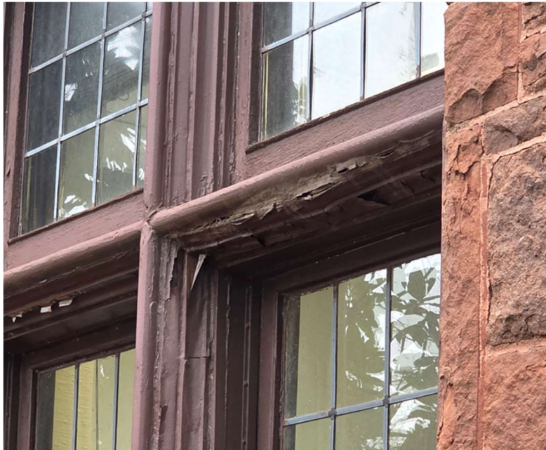
Photo 37: Egleston wood frame decay.
