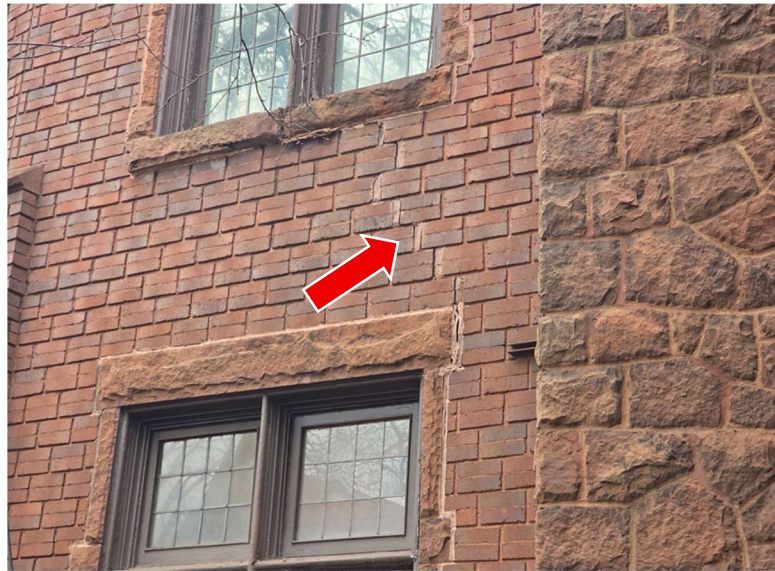
Photo 28: Egleston brick crack.
