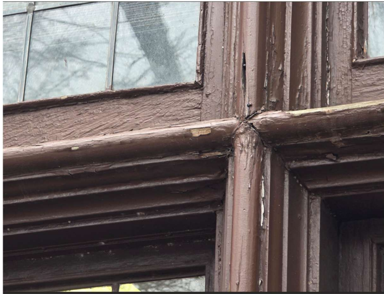
Photo 35: Egleston wood frame decay.
