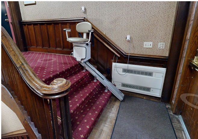
FIGURE 6 EXISTING STAIR CHAIR LIFT IS NOT COMPLIANT WITH ADA REQUIREMENTS
