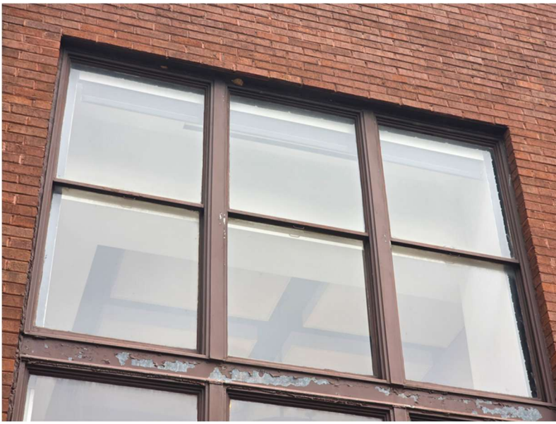
Photo 41: Parish Hall steel window with coating deterioration.
