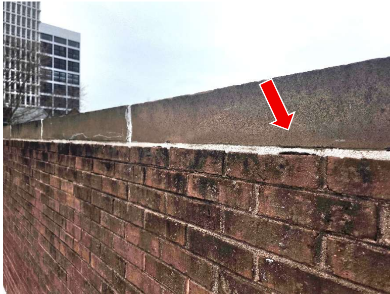
Photo 22: Parish parapet coping with open joint.
