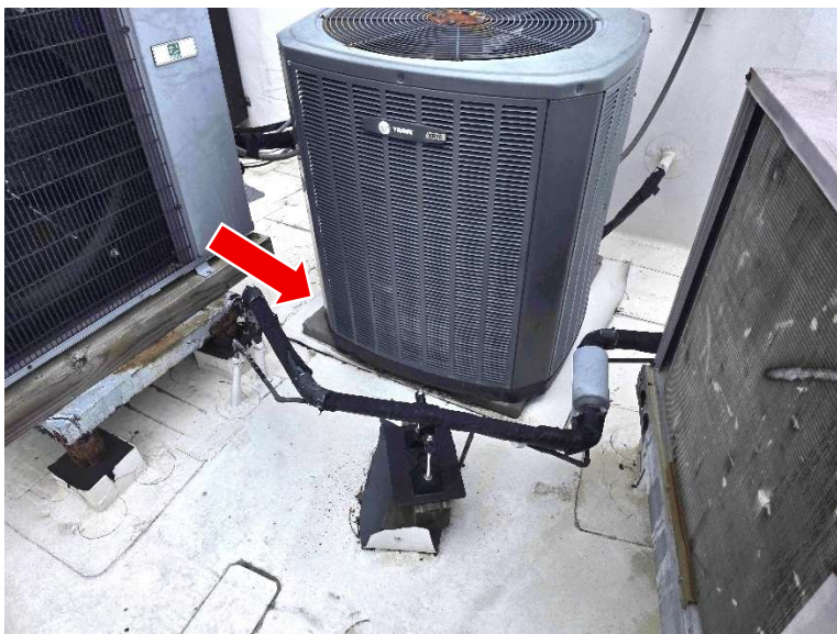
Photo 16: View of Egleston TPO roofing with mechanical unit lacking roofing curb.
