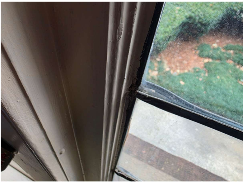
Photo 44: Egleston window lead came deformation.
